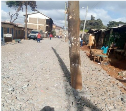
Figure 2: Just how are they going to tarmac the road (note the electricity pole)?
